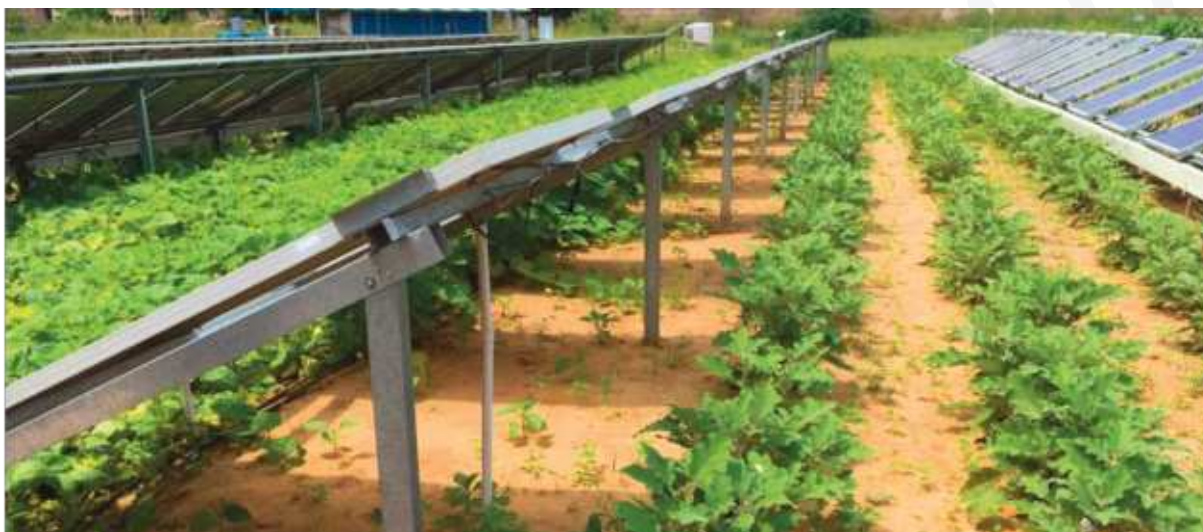
Central Arid-Zone Research Institute (CAZRI) Agrivoltaics plant, Jodhpur, Rajasthan. © CAZRI.
