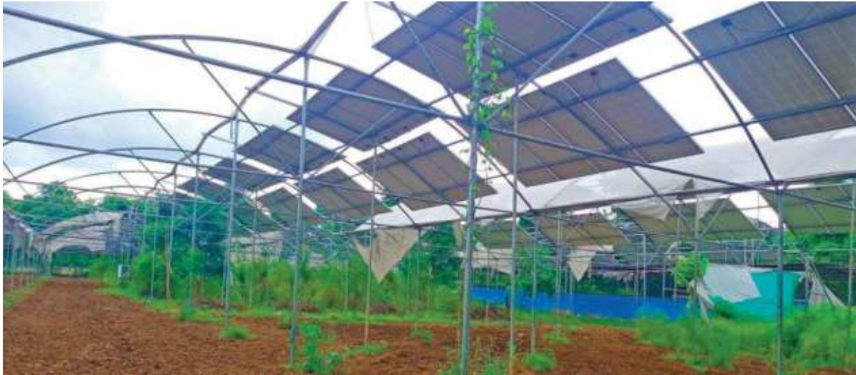
PV panels retrofitted onto a polyhouse. © Khare Energy Private Ltd.
