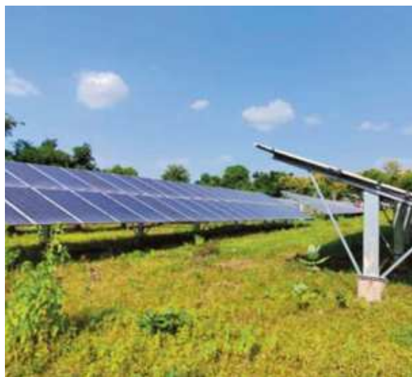
Plant A, Indra Solar Farm, Agrivoltaics plant, Tikamgarh, Madhya Pradesh. © Khare Energy Private
