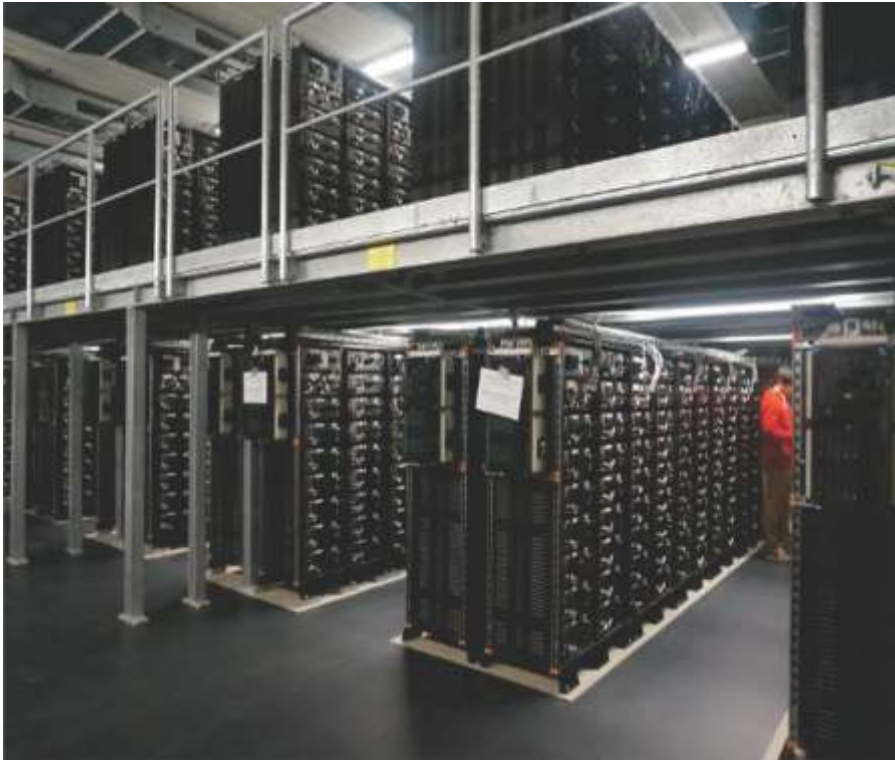
Relyon - Solar - Advanced - Battery - Storage
