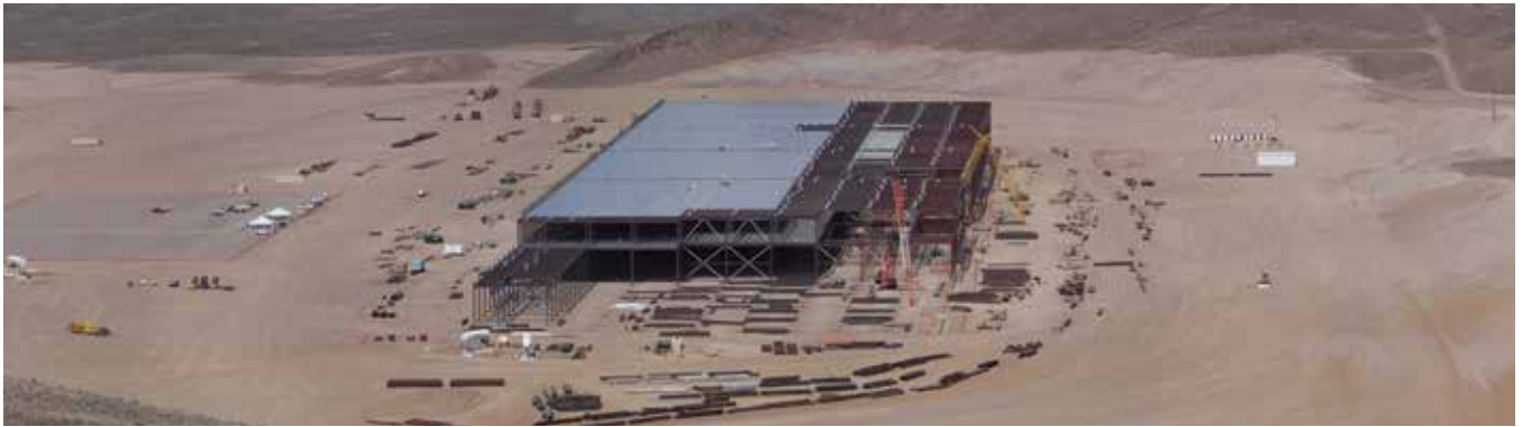
Aerial image of Tesla Gigafactory. Gigafactory construction progress 03.03.2015, as seen from the air. The finished building is 40%.
