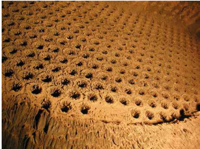
Figure 3: Heat exchanger similar to Figure 2 with major fouling and slag formation caused by the fly ash in the flue gas due to excessive temperatures (same effect as in Figure 1).
