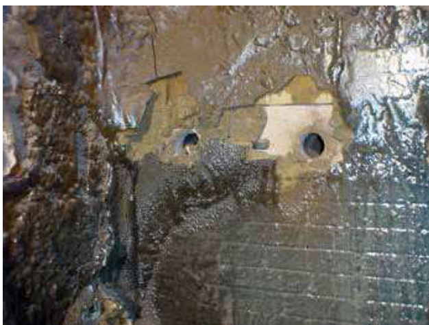
Figure 1. Slag formation in the combustion chamber of a wood-fired boiler caused by temperatures above the deformation temperature.
